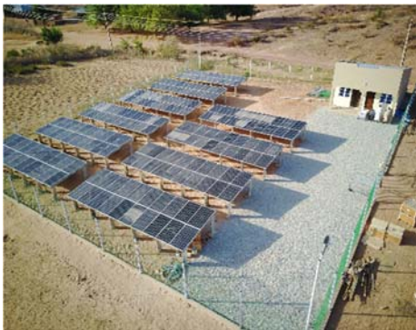
Aerial Vie of Commpleted 60kW Power Plant
